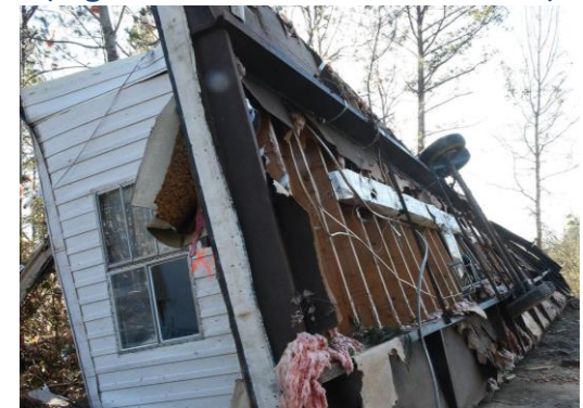
Wind Damage (e.g. recent tornado in Alabama)
